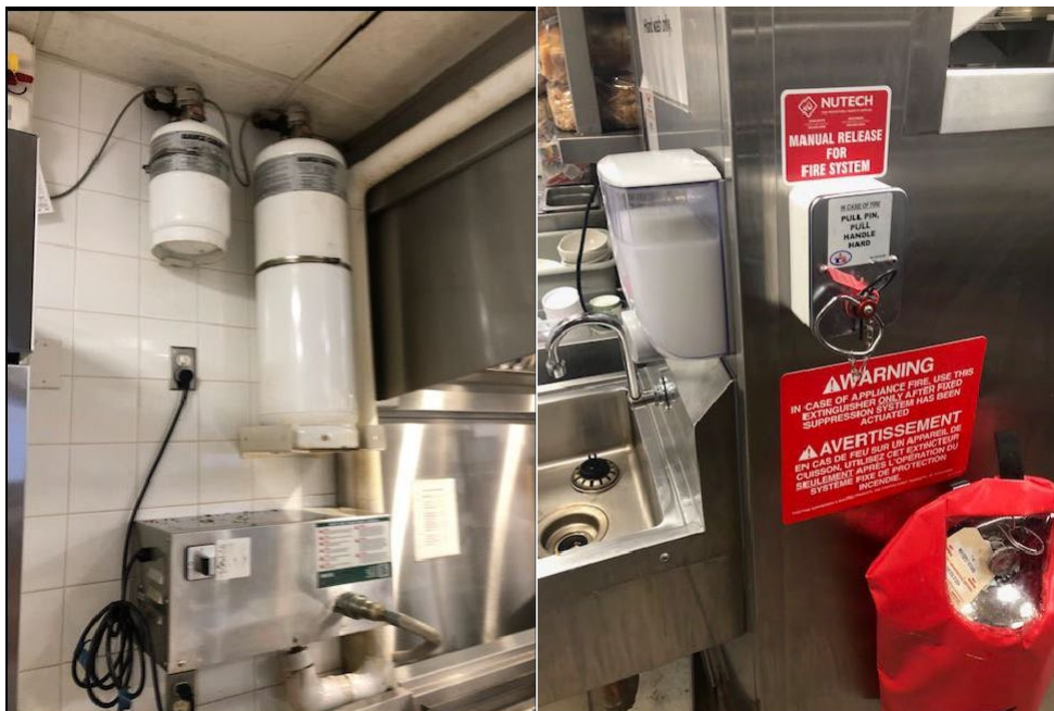
Kitchen Auto suppression system and Manual Activation device.
