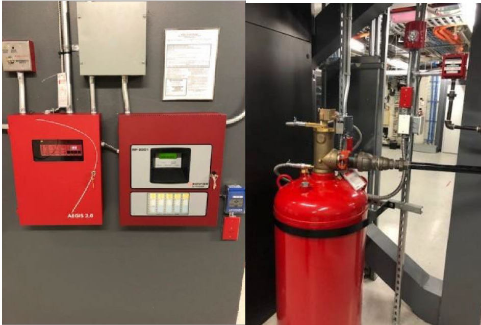
Novac 1230 Suppression system and controls in LAN Room
